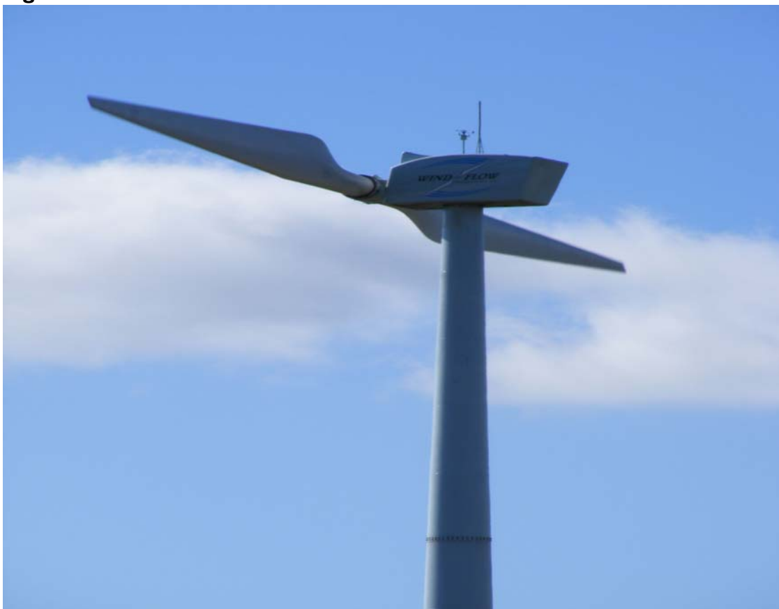
Figure A6.3 Windflow 500 Turbine
